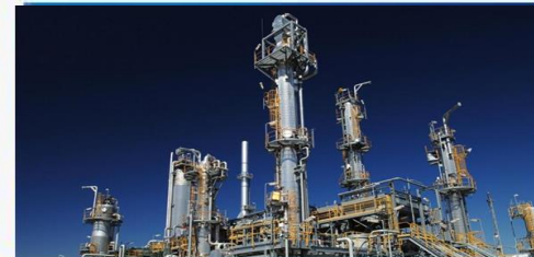
GAS PROCESSING PLANTS
