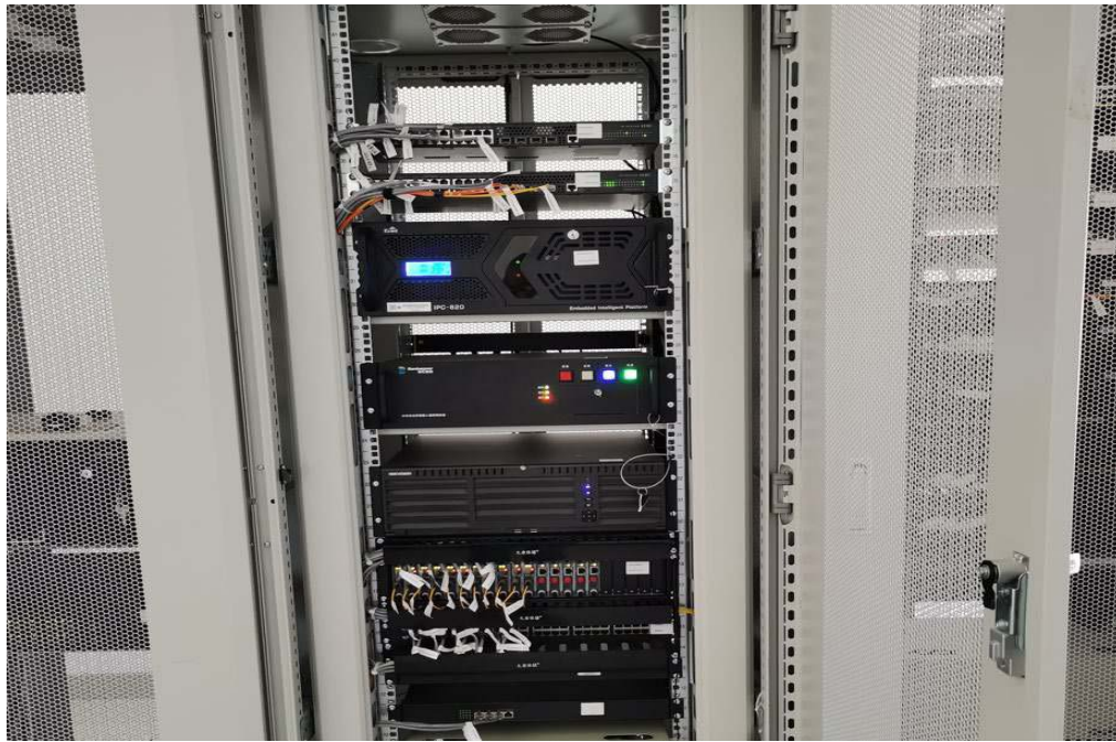
Figure 7 - FenceSentry 安裝在控制室
